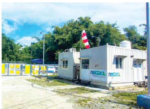
Mangaldoi CGS-Station Infrastructure
