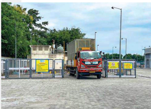
1 st CGS cum Mother Station of NEGDC at Tezpur
